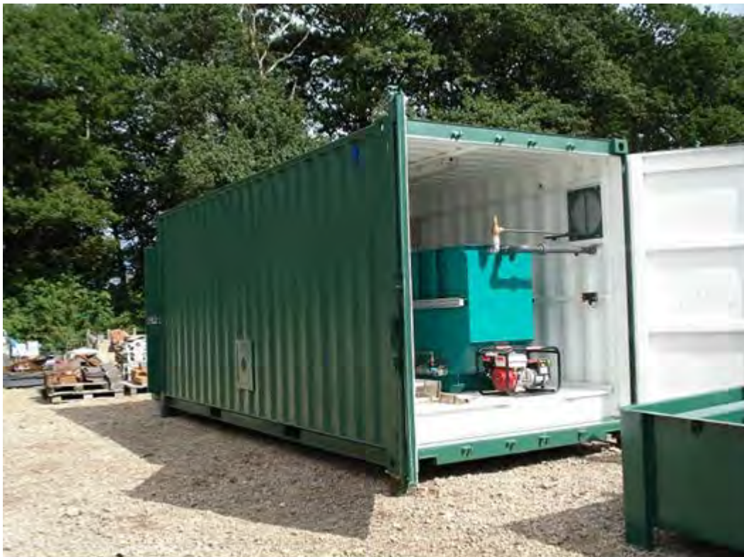
Figure 1 MFC pilot plant of the University of Nottingham
