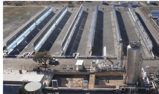
Figure 2. Top view of the TCP-100 field at Plataforma Solar de Almería (PSA-CIEMAT). The three loops are shown, with two PTCs in each of them, numbered from 1 (rightmost) to 6 (leftmost). The first loop is formed by the connected pair 1-2 (right loop), the second loop by 3-4 (center loop) and the third by 5-6 (left loop).
